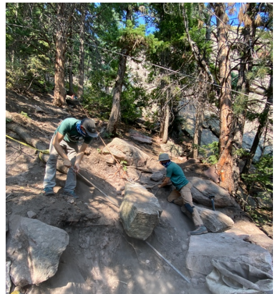
Figure 2: FRCS crew using a belay system to lower a large rock down onto the worksite.
