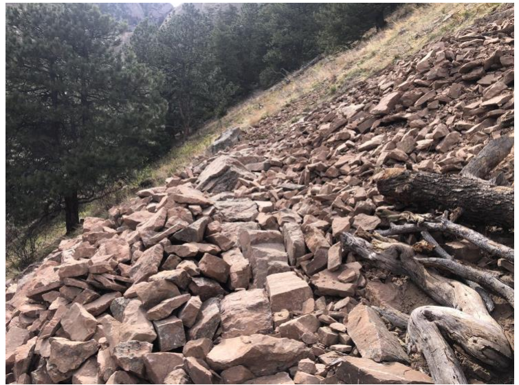
Figure 1: Paving stones were used to gain trail height versus a more traditional stone staircase.
