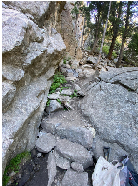
Figure 14: Belay pad with retaining structure built to protect the base of the popular Climbing Route Strange Science 11c. (Phase II)
