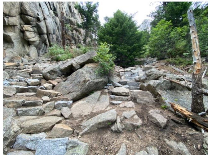
Figure 1- Construction of a primary path (Right) with an alternative path (Left) that leads to the climbs at Broken Rock.
