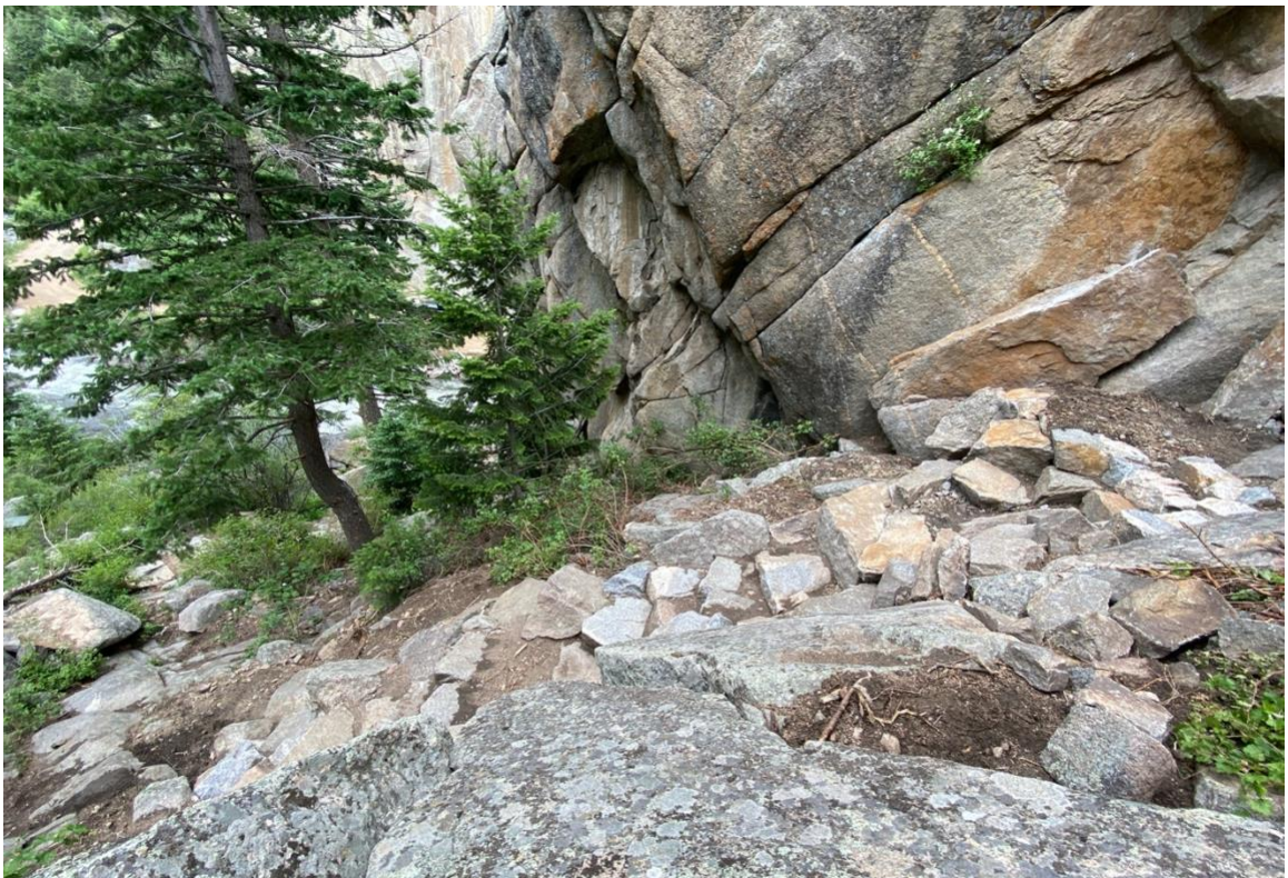
After: A stone staircase and retaining wall was constructed to provide clear access to the climbs in the area
