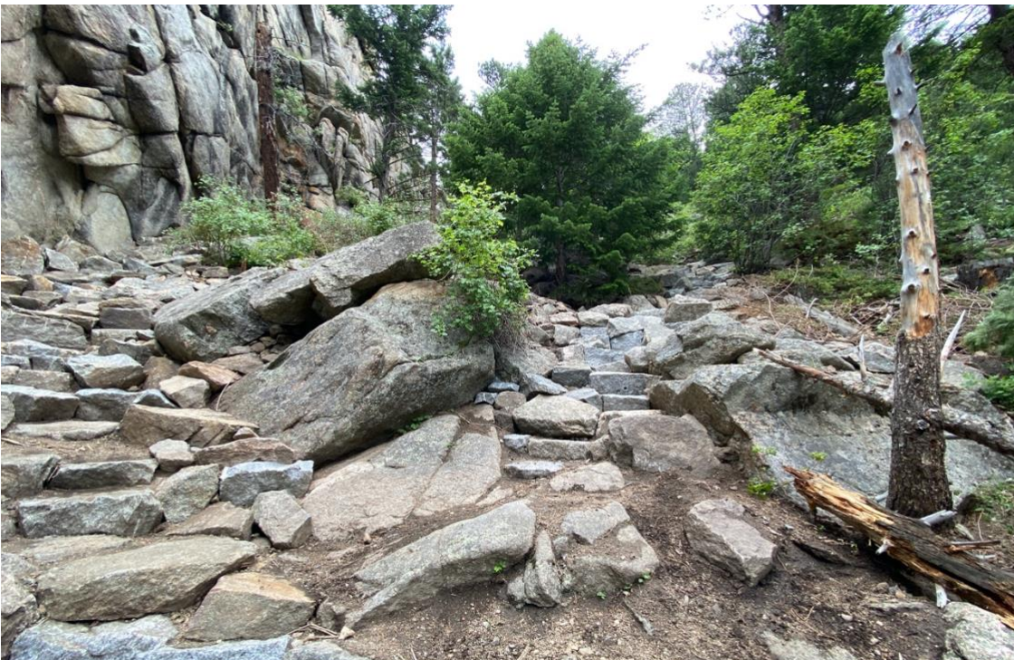
After: Stone was brought in and used to build a primary trail for all users while also providing an alternative for climbers to access the climbs on the left of the trail.
