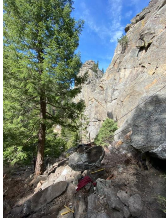
Figure 3- BCC staff utilized a high line rigging system to transport large amounts of stone to the build sites.
