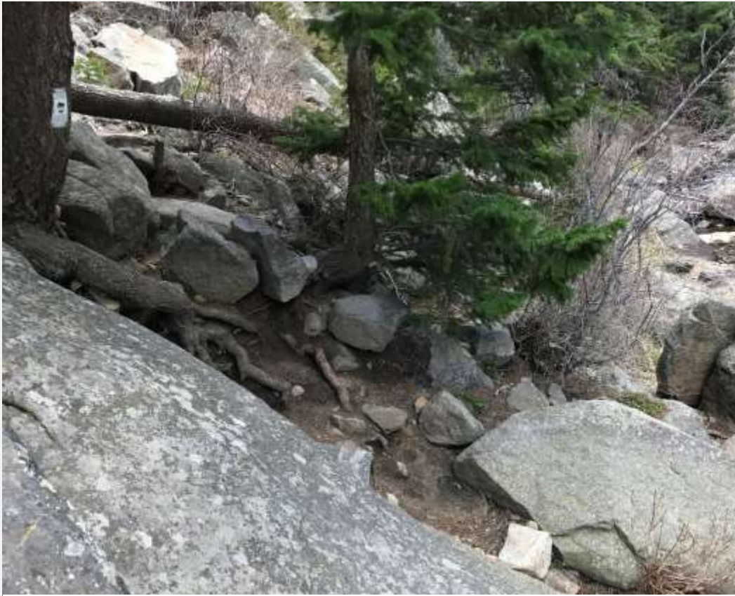
Eroded Trail/Streamside slope - Before
