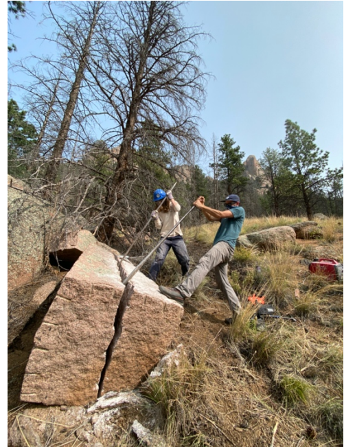
Figure 3: FRCS and ACE crew members working together to split stone which then had to be transported to the worksite.
