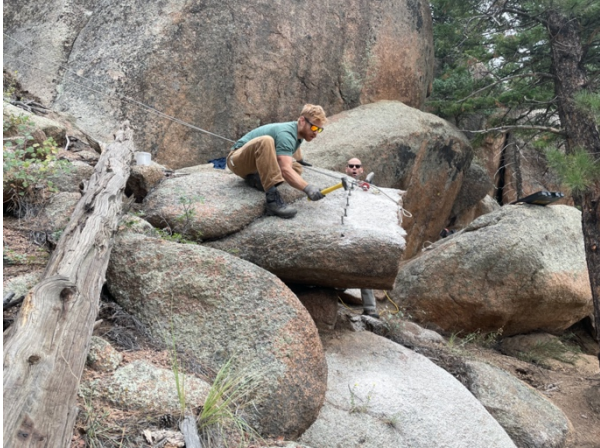
Figure 8: BCC crew member Nate showing a volunteer how to quarrying stone for a staircase (2022)
