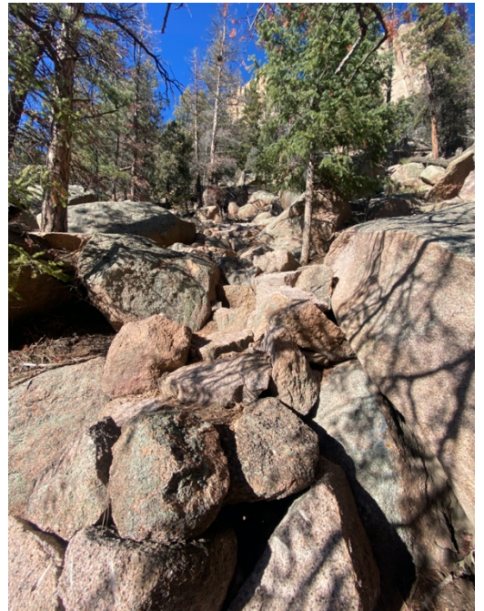
Figure 24: The first of three steep technical staircases built with stone steps and retaining structures at the location of Figure 23 After (2022)
