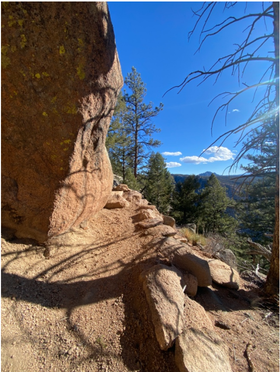
Figure 26: Trail constructed with retaining structure supporting tread in location of Figure 25 After (2022)
