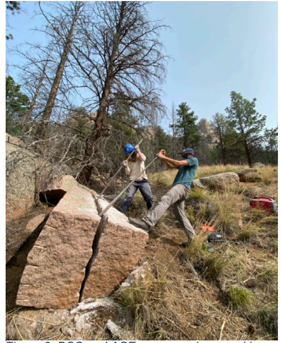
Figure 3: BCC and ACE crew members working together to split stone which then was transported by hand to the worksite (2020)
