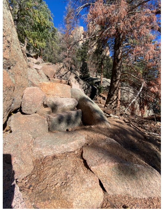
Figure 22: Building off of the work from 2020 beginning the first large staircase at the location of Figure 21 After (2022)
