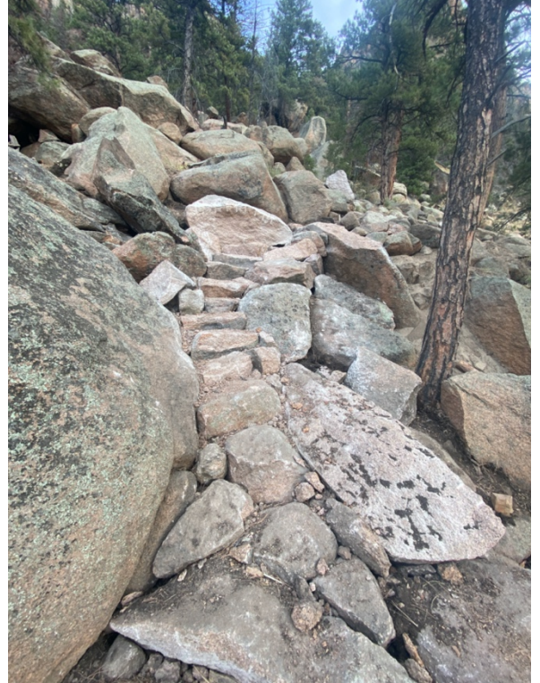
Figure 18: Large dead tree removed and replaced with large technical stone structures at location of Figure 17 After (2021)
