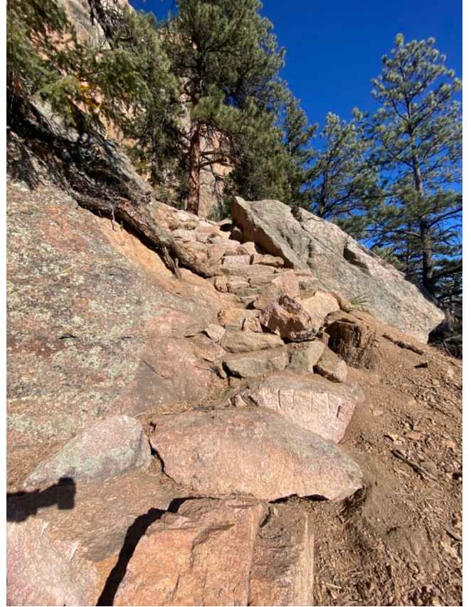
Figure 20: One of the BCC's more challenging builds of this project. Having to cut through a narrow gap of slab on the left and rock formations on the right at the location of Figure 19 . After (2022)
