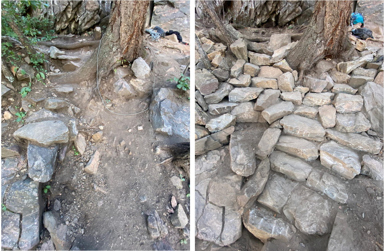
Figures 12 and 13: This is the highest trafficked area of the crag, which is the junction between the East Wall and main wall of Lower Tiers of Zion. The old eroding structure (left) was not built to withstand the traffic of the crag vs the new professionally built structure (right).
