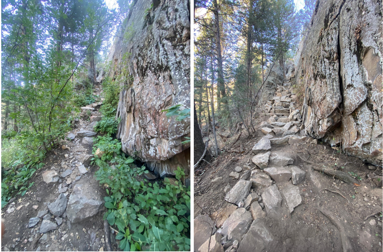
Figures 10 and 11: New stone staircase(right) leading to the East Wall of Lower Tiers of Zion. The Old gully (left) was full of loose rocks and was a major tripping hazard.
