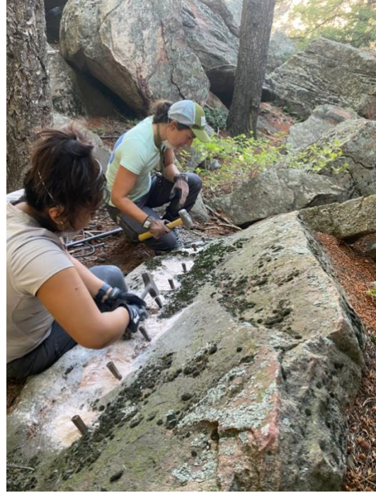
Figure 3- Quarrying was performed away from the site and then stones were transported to the worksite via a highline rigging system.
