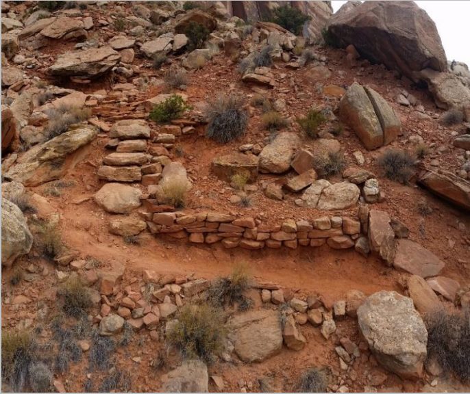
Before – eroded stairs & retaining structure
