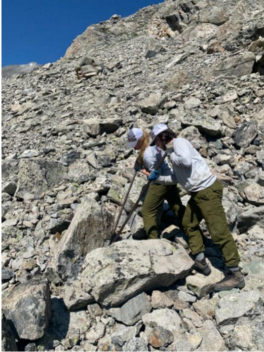
Figure 2: RMC crew members shifting larger stones that would eventually become the retaining structure for the built trail.
