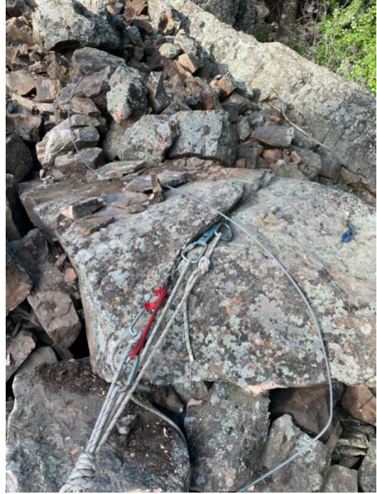
Figure 3- BCC staff utilized natural gear anchors to maneuver stone around while rigging.
