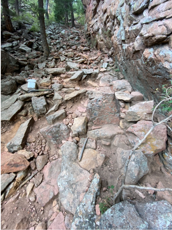
Figure 12: Another view of the unstable belay area under Unshackled 5.10+. Before
