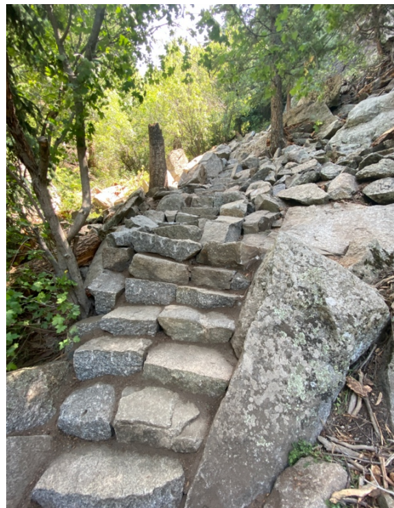
After: FRCS began construction directly on top of work from 2018 to continue the staircase leading into the talus field.
