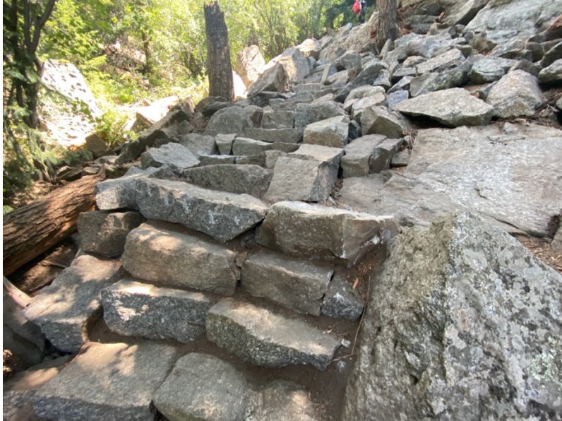
Figure 2- FRCS quarried locally sourced stone into suitable shapes to build staircases and retaining walls.
