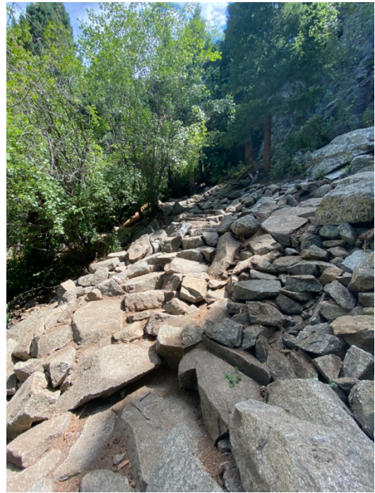
After: FRCS utilized the fallen trees for restoration and maneuvered stone in order to create a walking surface through the talus.
