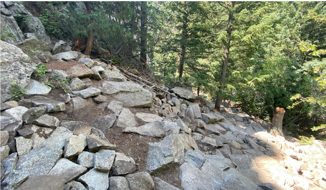
After: Heavy rock manipulation of the talus field provided enough space for FRCS to construct staircases and walking paths through the talus.
