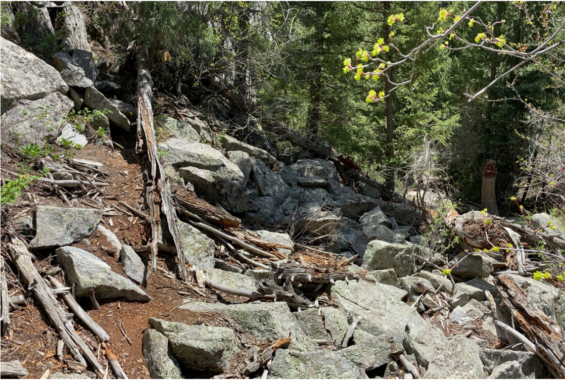
Before: The talus field in which the new rerouted trail is going to run through
